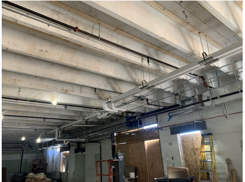
Area G - Overhead MEP systems
