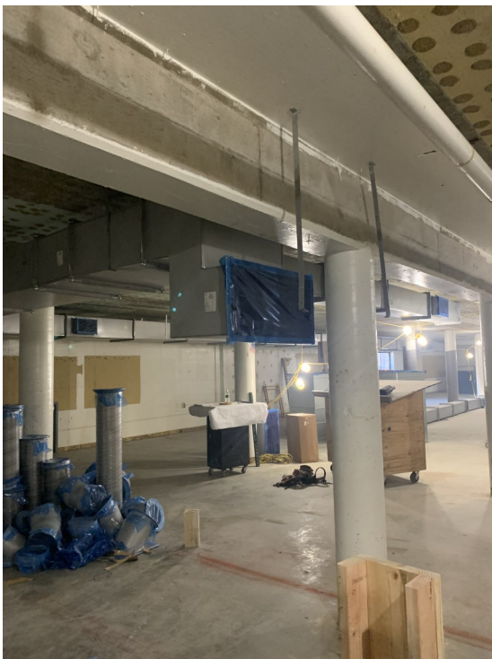
B Building Basement—Overhead Mechanical Ductwork
