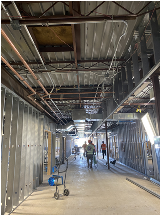
Area D - Level 2 - Wall and Ceiling Framing and Overhead Mechanical, Plumbing, and Electrical
