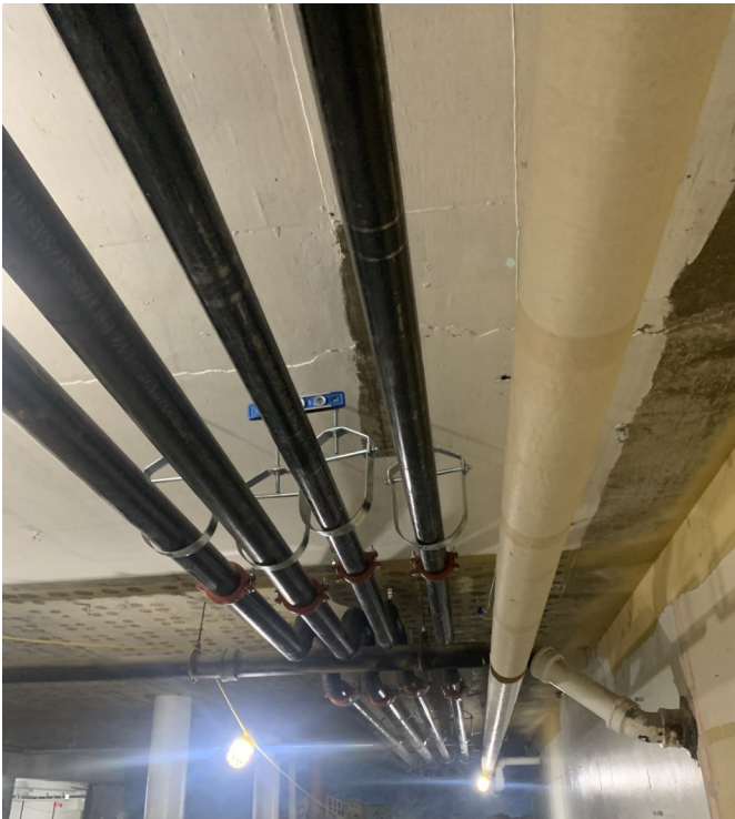
B Building Basement—Overhead Mechanical Piping
