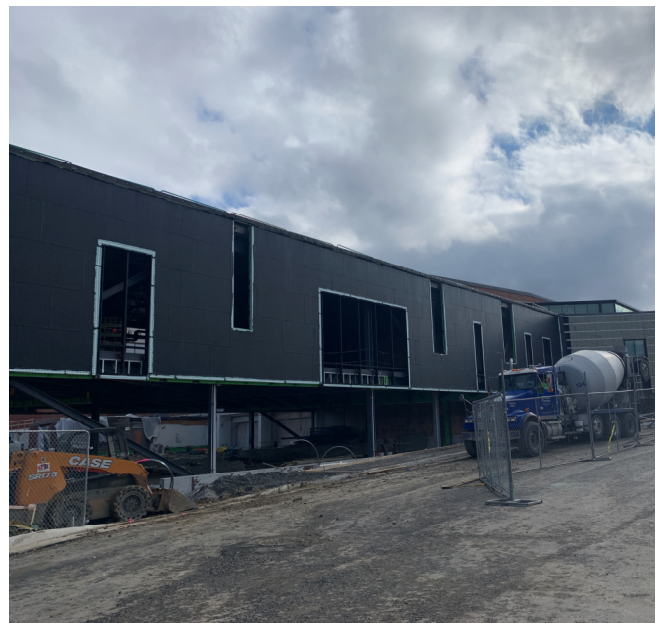
Zone C—Addition 2 North—West Side Skin
