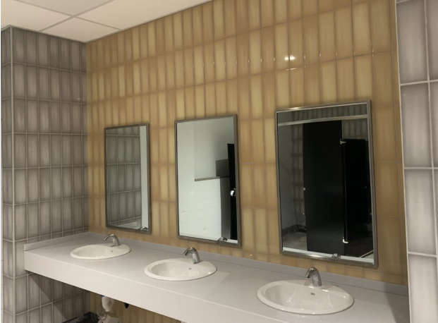
A Building - Tile, Countertops, and Sinks in Restrooms
