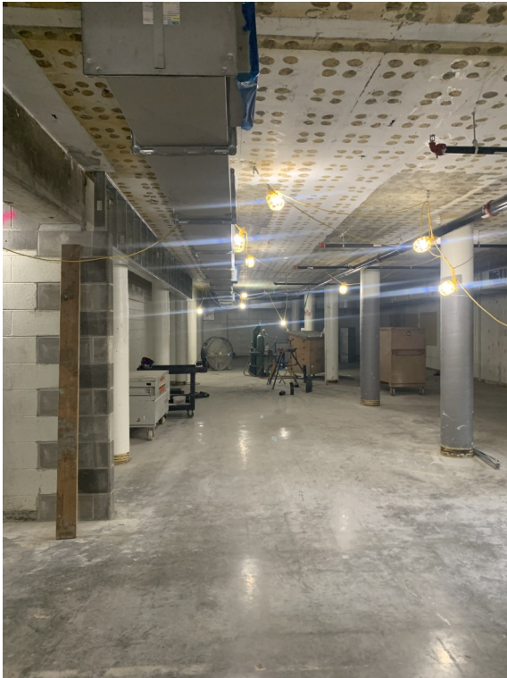
B Building Basement—Overhead Mechanical Ductwork in Teacher Collaboration
